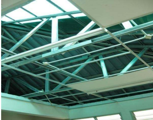
Gambar 3.9 Siling Tandas Rosak
